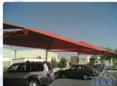
66 - Car parking shade. HDPE fabric
